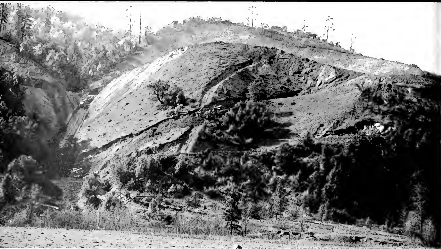
Equipment grading for relocation of State Highway (U. S. 99) through mountains north of Shasta Dam at south end of the Antler bridge across the Sacramento River in Shasta County. Abutment of bridge is seen at right of picture.
